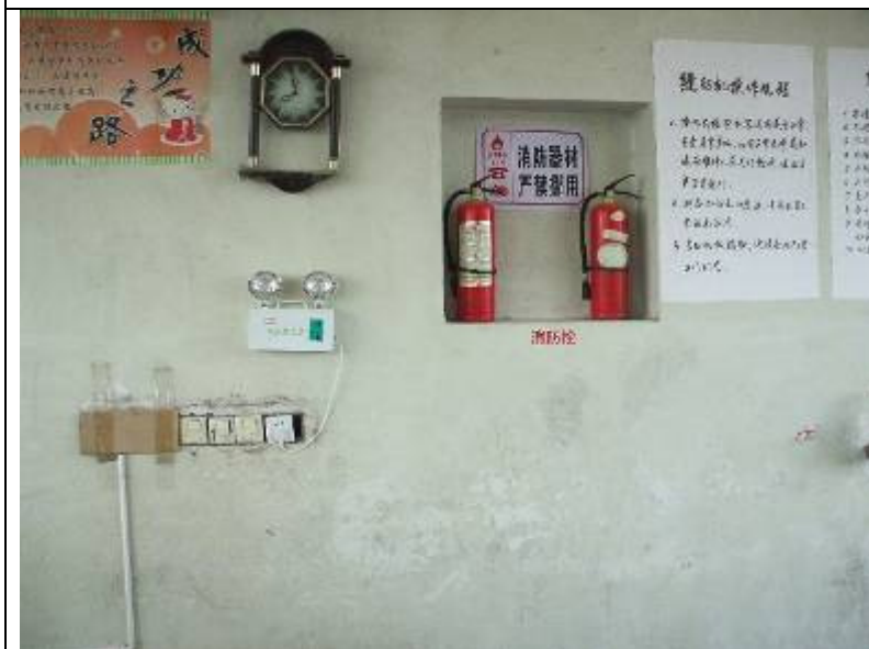
Fire extinguisher and exit sign
